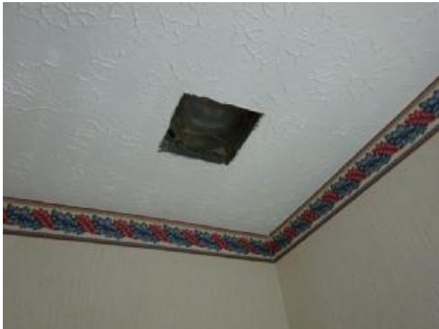
Missing vent cover in bathroom ceiling
