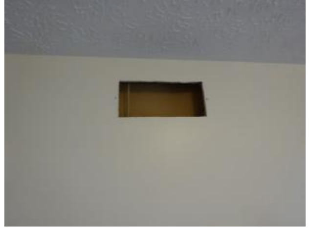
Missing vent in bedroom wall
