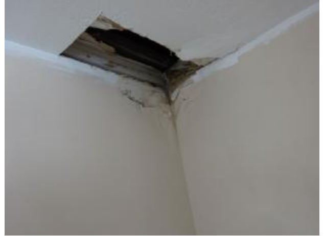
Water damage and missing vent in bathroom
