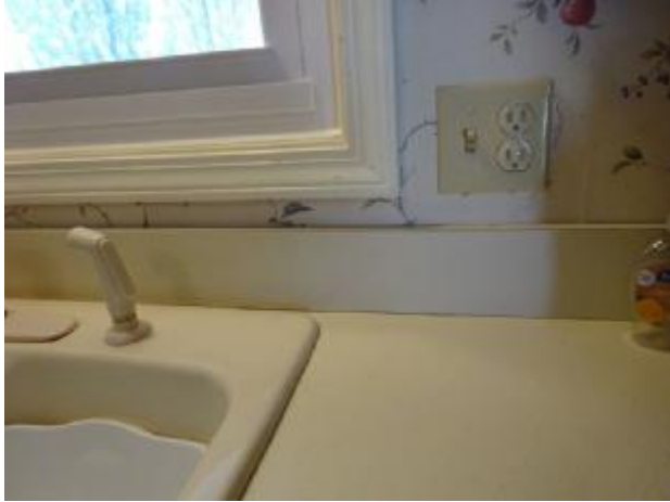
No GFCI by sink
