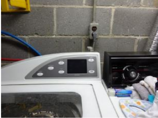
No GFCI outlet by washer
