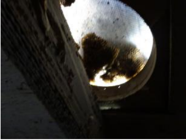
Wasp nest in roof vent
