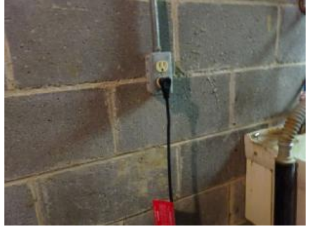
No GFCI outlet by sink
