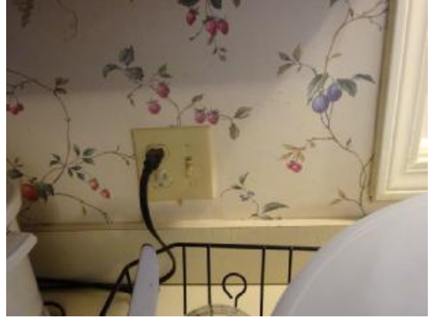
No GFCI by sink
