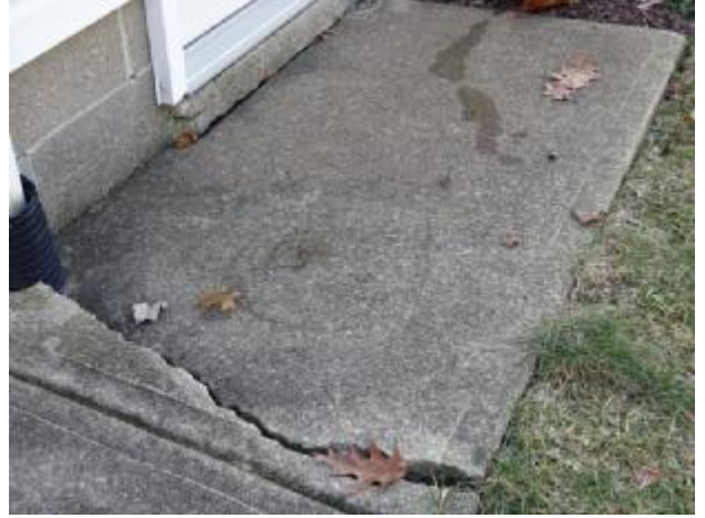
Slab by garage door sunk
