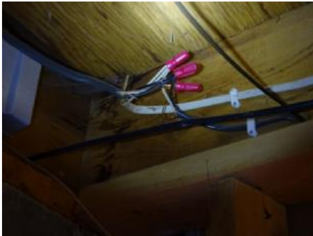
Exposed wire junction
