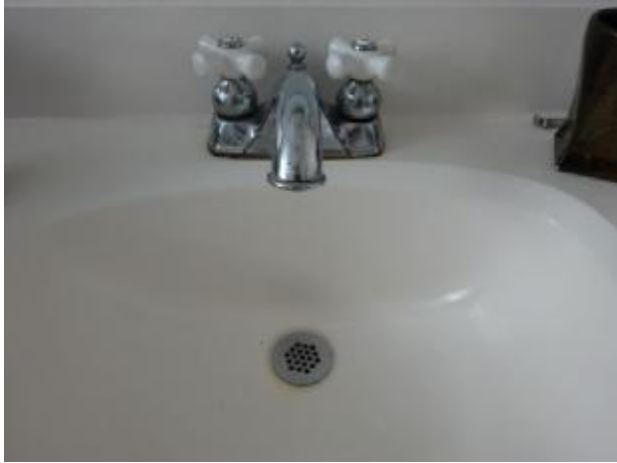
No stopper in downstairs bathroom sink
