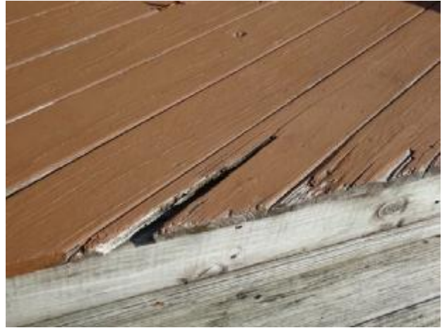
Deck floorboards rotted
